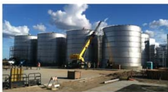
Wine Storage Tanks with Dimple Style Refrigeration Jackets Paso Robles Tank, Inc.
